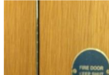
Obvious hazards include ... large gaps between fire doors
