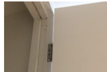
...fire door with missing smoke seals and intumescent strips, often incomplete or damaged
