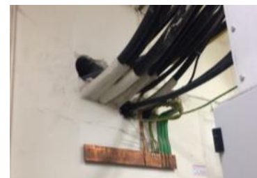
...breaches in the fire compartment requiring fire stopping work
