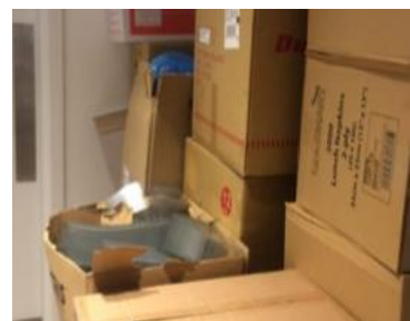
...excessive combustible materials (fire loading) stored on means of escape
